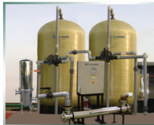
Water Treatment With Disinfection Plant
